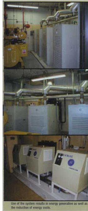
Use of the system results in energy generation as well as the reduction of energy costs.
